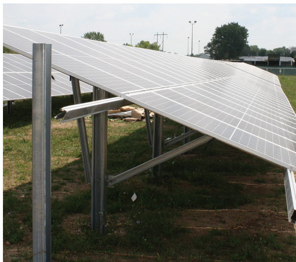
Construction on three new IMEA-commissioned solar photovoltaic units took place in the summer and fall of 2020.
