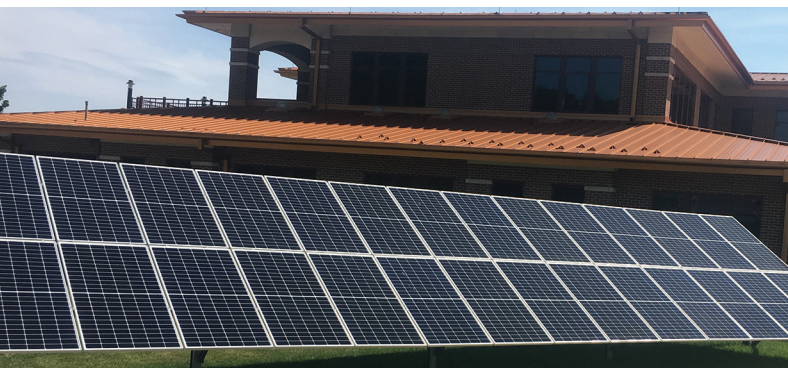
The new 10-kilowatt solar array at IMEA headquarters.
